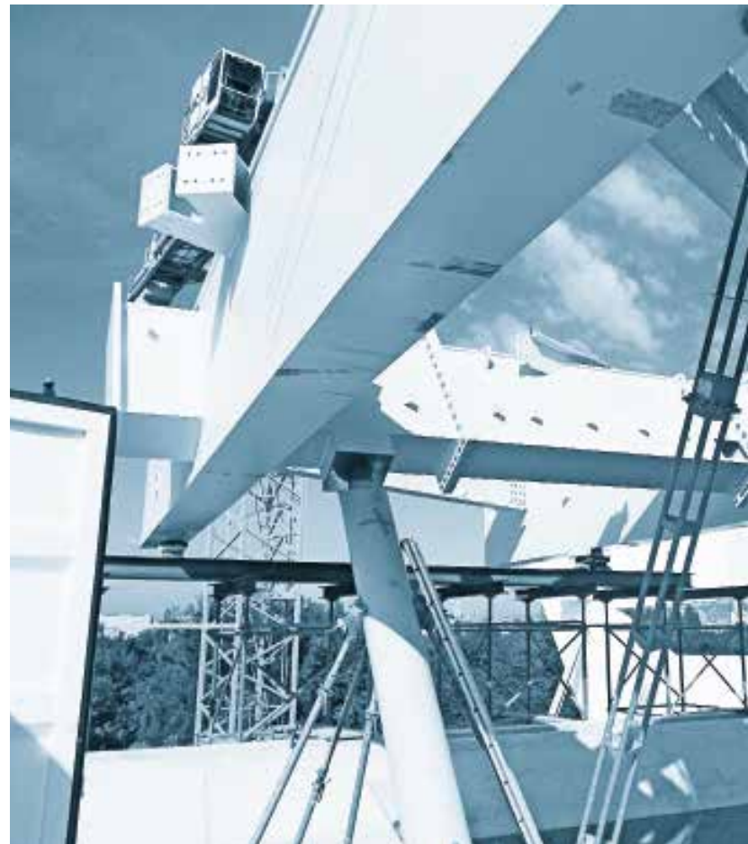
Library and Learning Center: Element des Hauptstahlfachwerkes Element of the main steel frame
